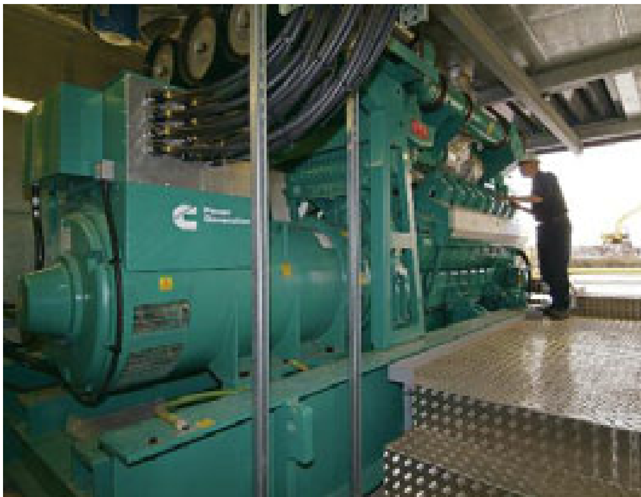
The new CHP plant started up in January 2008.
